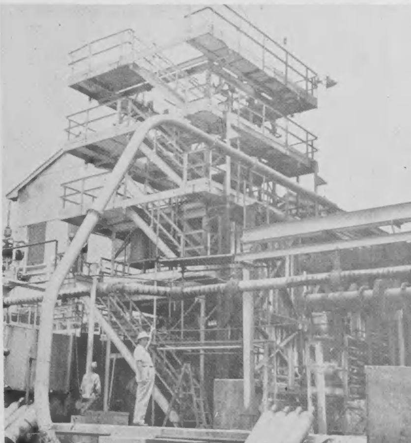
PROCESS VETERAN Lovelock Hassell (left) points to old SO2 Production Plant that is being dismantled. At right, simple tower and other equipment replaces old plant.
